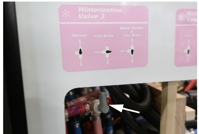
Winterization Valve #3 (Located on Water Center Panel shown in normal position). -Typical View
