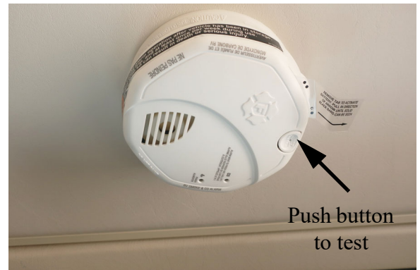
Smoke/carbon monoxide alarm. -Typical View
